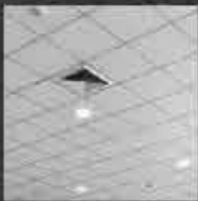
CEILING GRID FALSE CEILING
